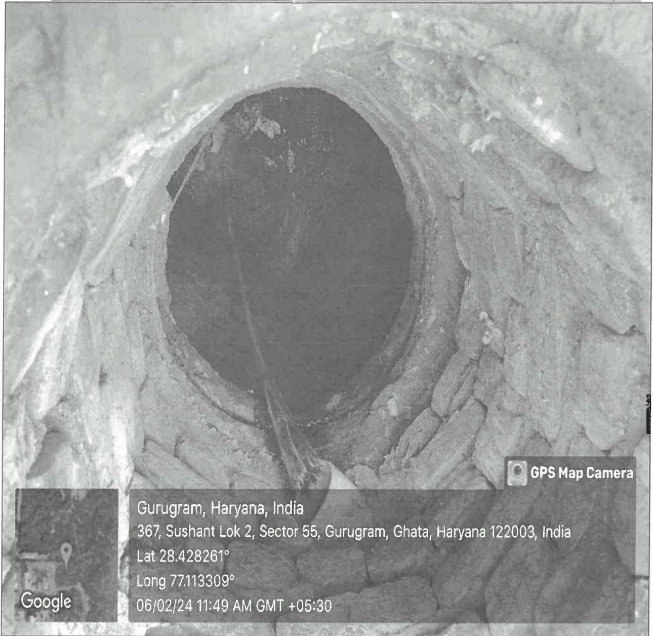
200KLD STP in Sushant University Campus
